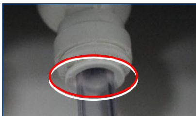
Fig. 51: Ring on drain valve
